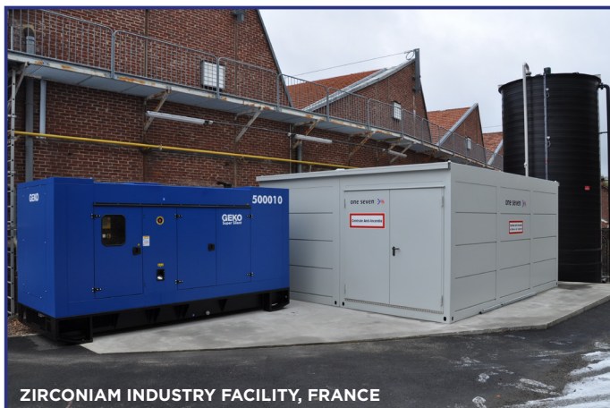
ONE SEVEN® STATIONARY SYSTEM INSTALLED IN CONTAINER OUTSIDE OF A FACILITY
